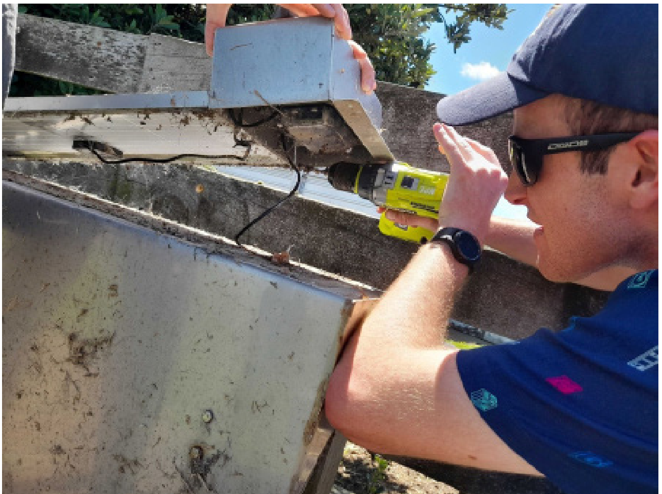
Levno Hardware Team Member Stanley Jackson installs Levno's water monitoring gear on a meter in one of the first sites in Sutherland Road Manaia.
